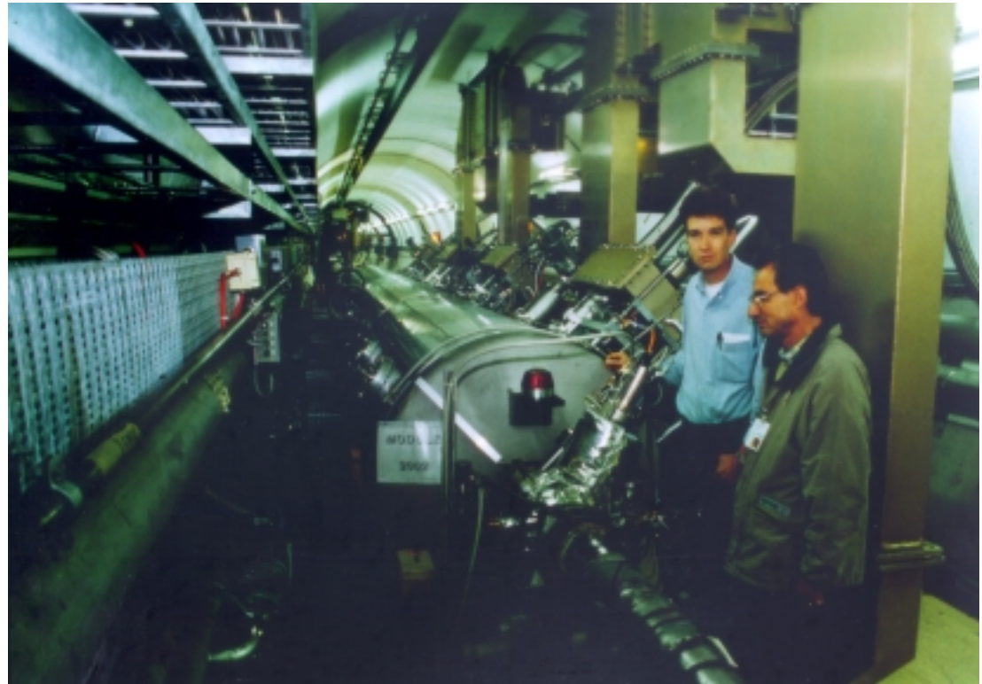
SC module installed in the LEP tunnel
